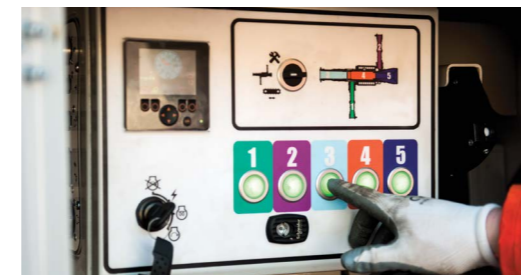
Colour coded control panel for ease of operation
